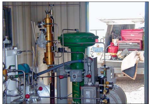
Figure 8.0 - Becker Flow Control Valve and Monitor
