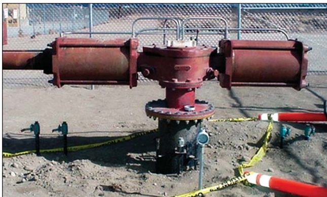
Figure 10.1 - Conversion of Existing On-Off Actuated Valve to Automated Flow Control (Before)
