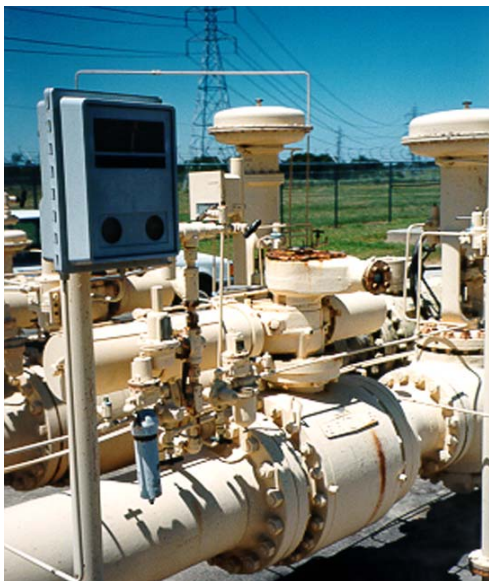
Figure 8.0 - Typical High Bleed Pneumatic "GAP" Controller (Before)
