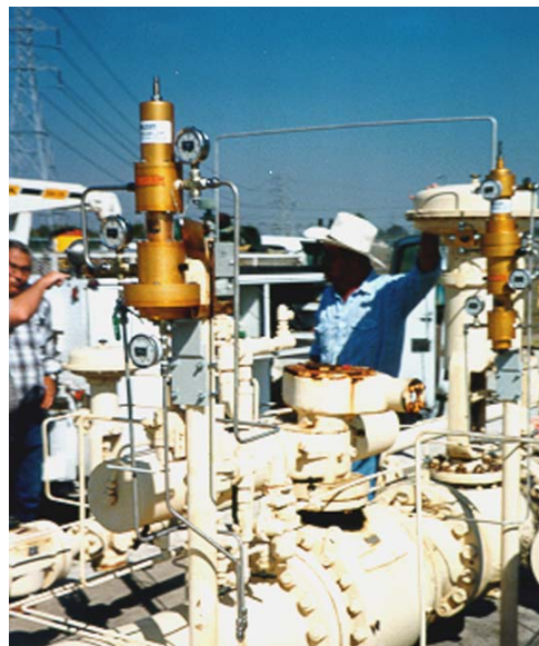
Figure 9.0 - Elimination of Constant Bleed Gas Emissions with Becker "GAP" Controller (After)
