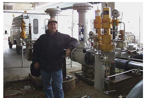
Figure 15.0 - Becker GAP Controller Provides Additional Protection Becker Globe Type Control Valves are equipped with VRP-SB Pressure Controllers to regulate flames in above photo. In the event of underpressure, a Becker VRP-SB-GAP Gap Controller will override and shut down the fuel feed until manually reset by qualified technicians.
