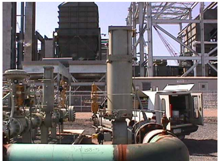
Figure 13.0 - Slam Shut Valve Installed in Natural Gas-Fired Power Plant Fuel Gas Feed
