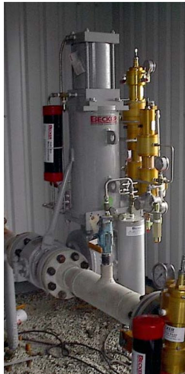
Figure 12.0 - Power Plant Fuel Gas Feed "Slam Shut" Override
