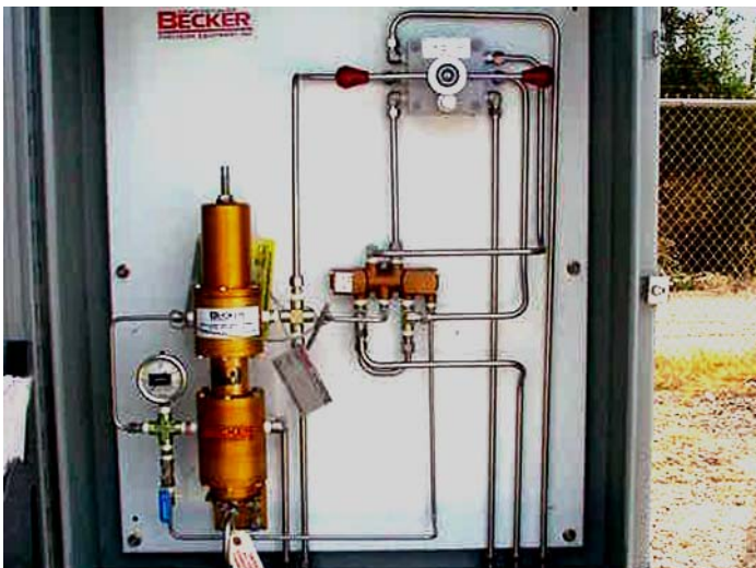
Figure 11.0 - Becker VRP-SB-GAP Gap Controller Installed in Cabinet Enclosure
