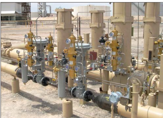
Figure 10.0 - Becker Designed Combustion Turbine Power Plant Fuel Gas Station
